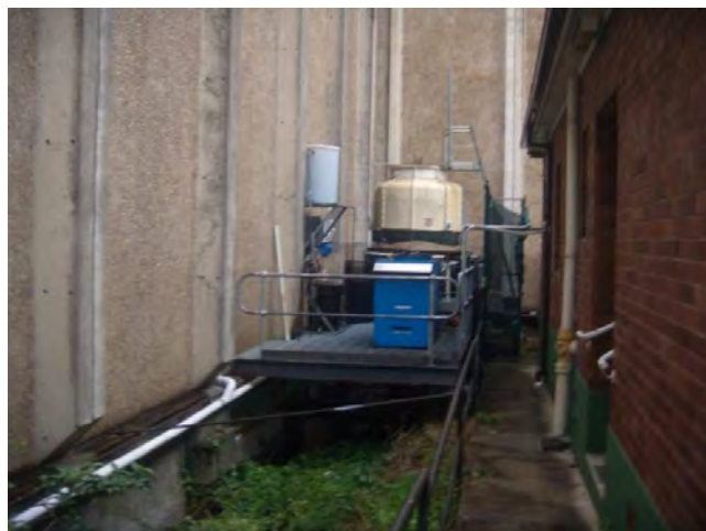
Site Photograph 5: cooling tower located between the warehouse and office in Lot 1 DP 599502
